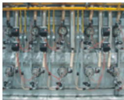
Roller hearth furnace
