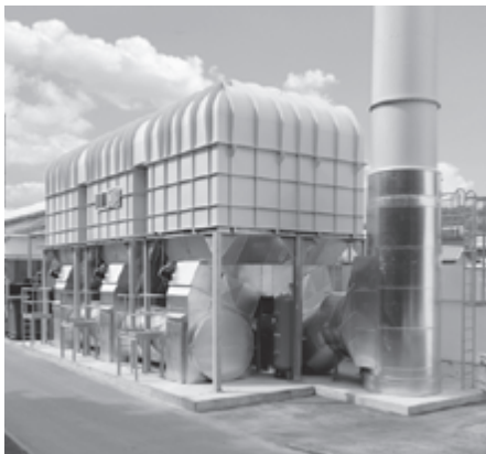
Incineration installation for thermal regenerative flue air purification
