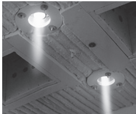
Overhead firing with burner BIC
